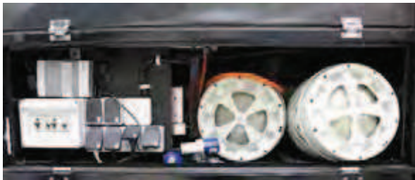
Figure 22: Old gas installation
